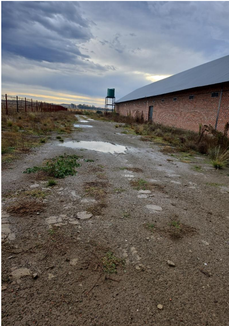
Figure 9: View looking south alongside the eastern layer house. The surface is a thin gravel and sand apron over compacted substrate. GPS (EXIF): 29.465727°S, 25.995042°E (29°27'56.62"S, 25°59'42.15"E); Field assessment: 5 May 2026, Banzai Environmental).
